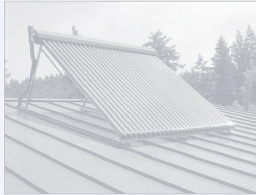
Solar Hot Water
