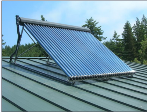
Solar Hot Water
