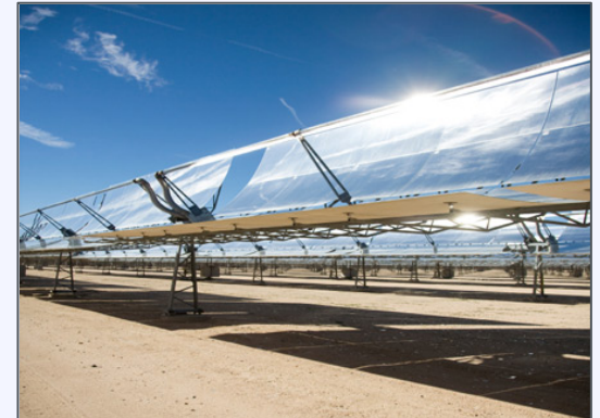
Concentrated Solar Power
