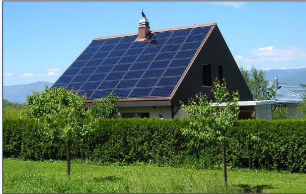
Solar Photovoltaic (PV)
